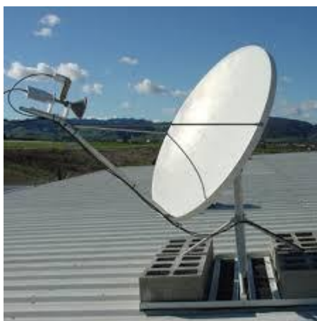
Figure (2): VSAT dish .
